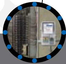
Whole home surge protection
