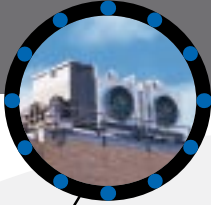
HVAC energy controls
